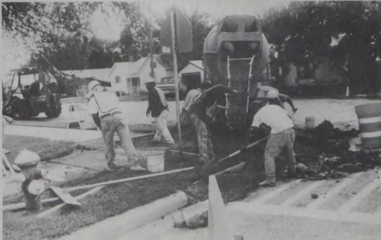
A DISTRICT-WIDE PROJECT of the Texas Highway Department is in progress in Muenster. Due to the American Disability Act that goes into effect in 1995, wheelchair ramps are being built on Hwy. 82 and Main Street, wherever there is a sidewalk along the street. Janie Hartman Photo
