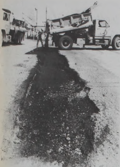
HIGHWAY DEPARTMENT WORKERS have been rerouting Hwy. 82 traffic in Muenster this past week, repairing the subgrade and base on the road. A rubberized seal with a new hot mix overlay will improve the roadway from the east side of town to Maple Street. Starting in July, the department will repave Hwy. 82 from Muenster to Saint Jo.
