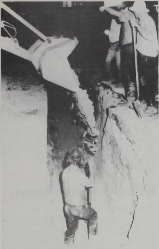
CITY EMPLOYEES put in late hours relocating a water main under Highway 82 Monday night. The move is necessary to accommodate the future installation of a storm drain by the Texas Highway Department. David Dittfurth is spreading sand in the trench. Tony Hess and Chris Yosten are above. Hermie Grewing is dumping sand. The pipe was moved from 5 feet deep to about 9 feet deep. Dave Fette Photo
