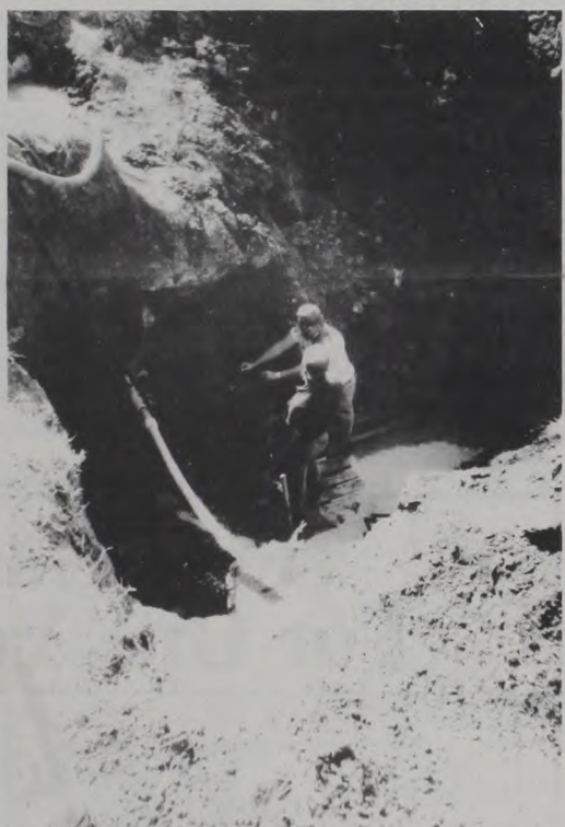
WORKERS drill a four-inch pipe 11 feet under Hwy. 82 at the intersection at Walnut Street to bury telephone cables. The Highway Department plans to rechannel runoff water and reconstruct the storm sewer in that vicinity in the near future. Additional details on the project will follow in The Enterprise when available.
