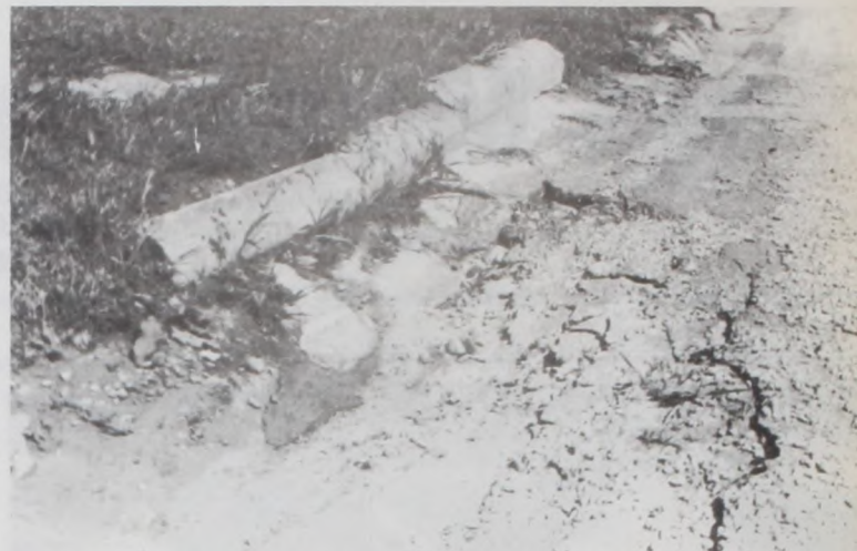
THE CURB on North Main Street won this week's Groad Hole Award. The broken, disappearing and unattended cement curb pieces clutter the edges of a sinking, unrepaired traffic land.
