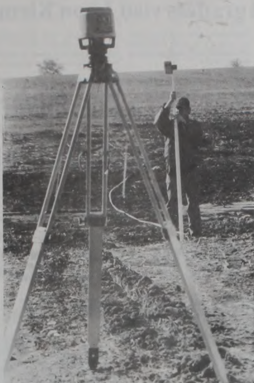
CONSERVATIONIST measures terraces constructed on the Ken Klement farm last fall. Janie Hartman Photo
