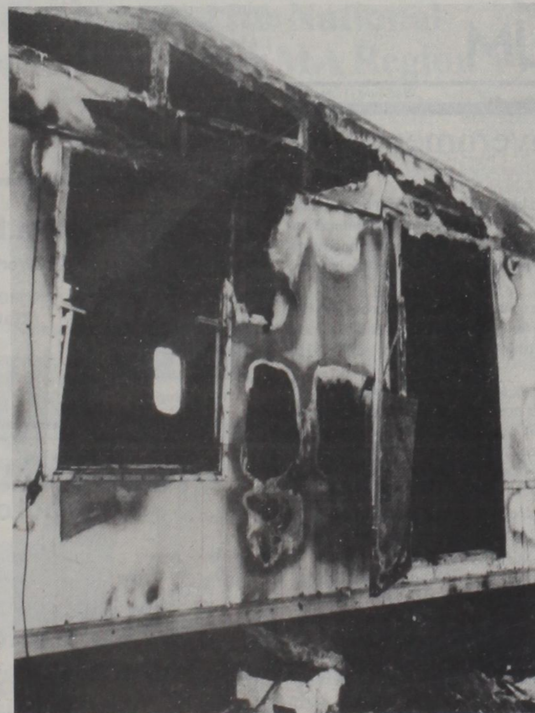
FIRE GUTTED the trailer home of Billy and Sandy Harris early Monday morning.
