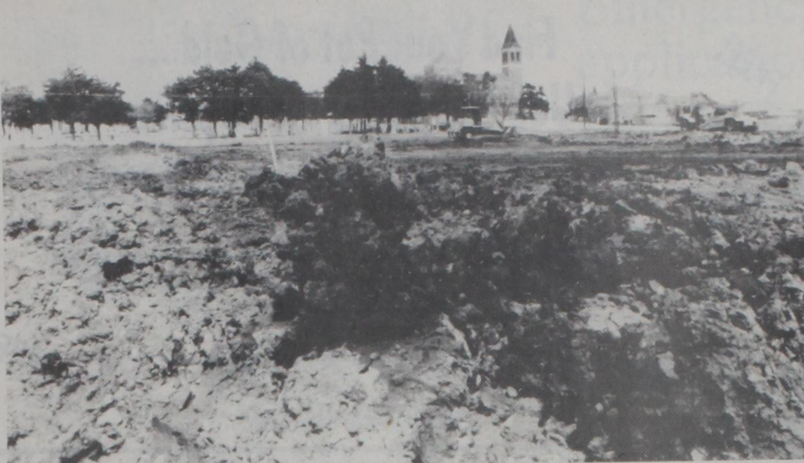
WORK CONTINUES, as the ground is prepared for the foundation of Lindsay's new parish hall and family center to be located just southwest of the parish grounds. Janie Hartman Photo
