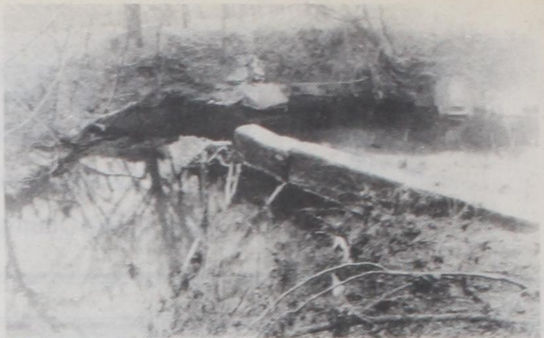
INSTALLED IN 1926 to pool water in a section of the Brushy Elm Creek in the Muenster City Park, this concrete barrier has buckled and cracked up during years past. It is retarding the flow of water through the park, causing the erosion of the creek bank's north side. Valuable park soil is being carried downstream and several trees will soon be endangered. The purpose of the barrier was to cause a collection of water for use in steam boiler drilling rigs on the west side of town. This area was brought to The Muenster Enterprise's attention by a concerned citizen who heard of the Park Pride Clean-up Project.
