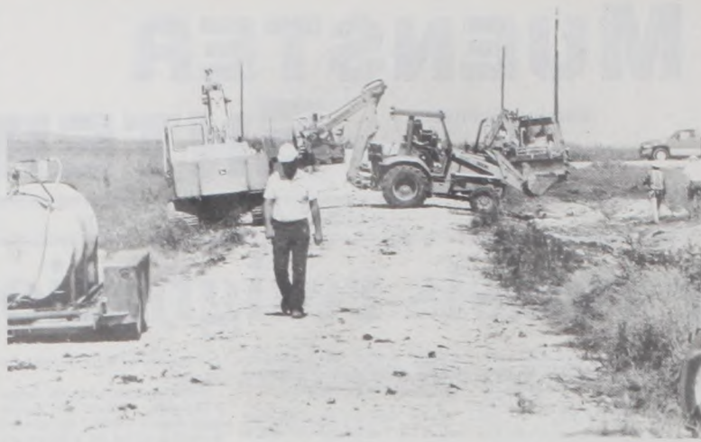
LINES ARE BEING BURIED north of Muenster to install fiber-optic cable. Muenster Telephone Corporation also installed telephone and cable television service to the Cler Acres Subdivision on FM373. The construction created a great deal of activity Tuesday afternoon on Alvin Road. Janie Hartman Photo
