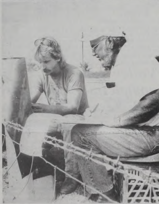
RODNEY DEXTER and Mel Chandler test telephone cable north of Muenster Wednesday for Mullens Cable Splicing of Little Elm.
