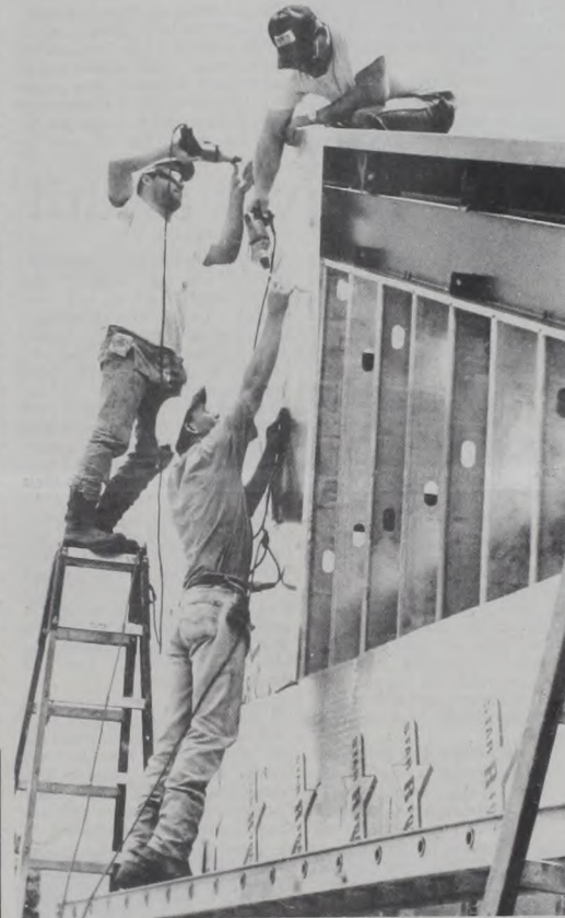
SHAWN, MARK and DAVID JR. FLUSCHE continue work on the 1400-square-foot addition to the Tender Loving Care Day Care Center of Muenster. The two rooms will be used for a 3- and 4-year-old Preschool that will begin in August and for after-school students for the day care.
