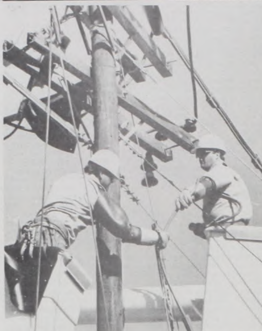
NICK WALTERSCHEID, left, and Floyd Haverkamp are both linemen for the Cooke County Electric Co-op. Both started as groundmen, then trainer and 3rd class linemen before earning their present position. Haverkamp has been at the Co-op six years and is a 1st class linemen, while Walterscheid began five years ago and has the 2nd class rank. The crew was replacing a pole and cross arms on a 3-way line split last week south of Muenster.
