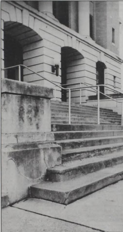
SINKING GROUND IS THOUGHT TO BE THE CAUSE OF severe damage to the east side of the historic Cooke County Courthouse. Crumbling steps, cracked foundation and other damage continues to worsen. Commissioners hope to be able to start repair work soon after consulting with the county's engineering firm, Komatsu. Photo by Dave Fette
