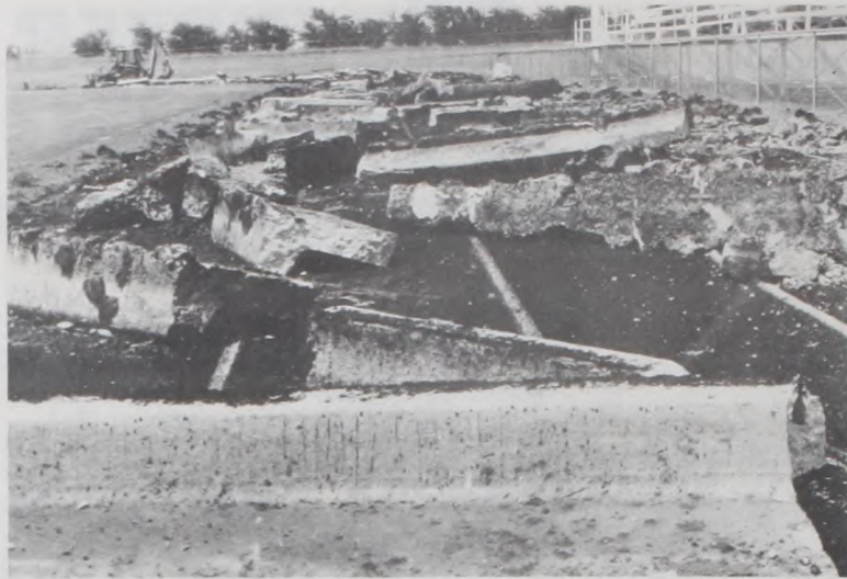
WORK CONTINUED on the Muenster ISD track Monday morning with the removal of the concrete curbing. Janie Hartman Photo
