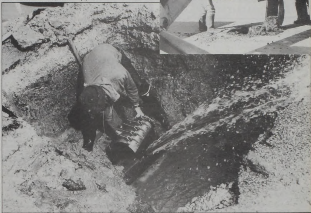
THE CITY OF MUENSTER has had its share of water problems the last weeks. Several valve leaks and three water line breaks have kept city workers busy. In the top photo, David Dittfurth (above) put on a clamp to fix the major break. Another major repair to a main water line Tuesday was on the 300 block of Main Street.
