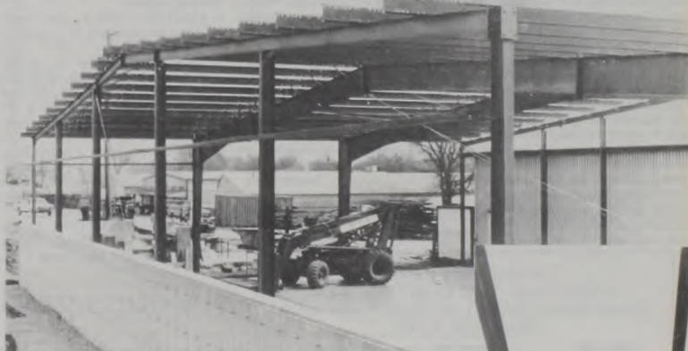
CONSTRUCTION CONTINUES at Flusche Enterprises, Inc. in Muenster. The expansion of the business includes a 60'x100' enlarged work area and a 30 square foot office. David Flusche, Jr. and Shawn Flusche work on the frame of the building. Staff photos
