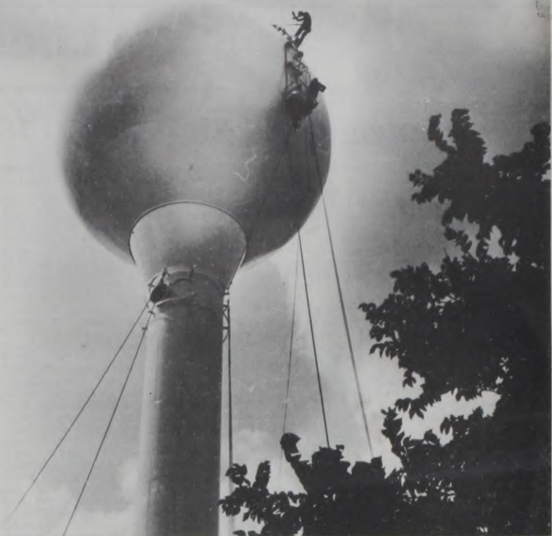
THE NEW LINDSAY WATER TOWER has received a series of protective coatings, inside and out. After the intermediate white epoxy coats and final white urethane have cured for 10 days "Lindsay Knights" will be painted on in five foot Gothic letters. The 30 day job has been done by Blue Ribbon Lining and Painting of Houston by the team of Tunney Bayles, Ed McGinnis, David Rowe, and Ryan Coffelt. Bayles estimates the paint job should last at least 10 to 15 years. The work included finishing many of the welded joints. The outside paint was applied with rollers to avoid waste and spray drift. Photo by Dave Fette
