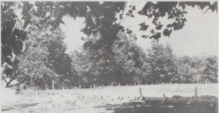
Established trees and landscape await the arrival of the new home for Chas and Carolyn Bayer. The sand and boards are set and ready for the cement foundation. Janie Hartman Photo
