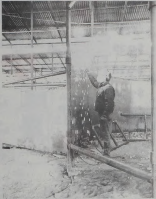
Welders construct solid steel walls in the holding pen and alley for better cattle management. Janie Hartman Photo
