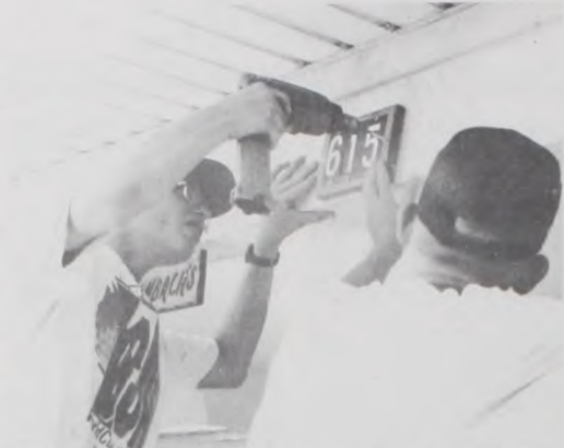
ROYCE AND ERIC KNABE are attaching reflective house number on the home of Mr. and Mrs. Tony Trubench, Jr. Fifty-nine homes of senior citizens received three-inch reflective numbers as Royce completed his Eagle Scout service project recently.
