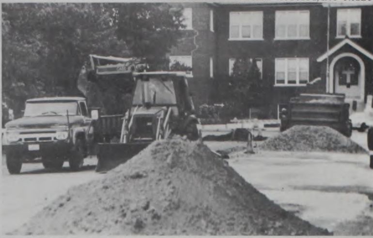
THE CITY CREW replaced a portion of Muenster's water line earlier this week. Work was being done on Oak Street in front of Sacred Heart School.
