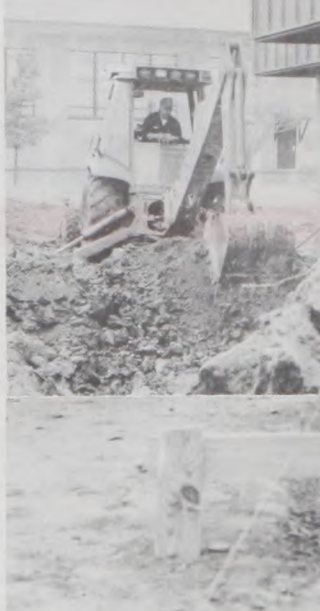
Dirtwork continues at the construction site of the new Muenster High School. At left, Bernard Hesse of G&H Backhoe works at the future front entrance of the school. Below, John Chizmadia, of Oden Mechanical Contractors of Wichita Falls, marks the location to be dug out for water lines going to the future home economics class room. Janie Hartman Photo
