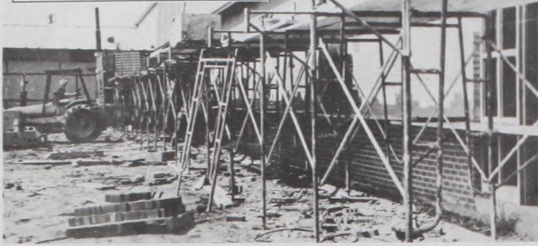
Progress continues at the construction site of the new Muenster High School building. Workers are attempting to complete the project in time to begin the 1999-2000 school year in the new classrooms, but are still several weeks behind schedule. Photo by Janie Hartman
