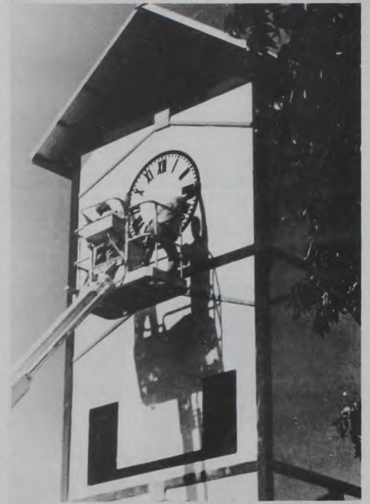
The Fischer's Market clock tower took another step toward completion this week with installation of the clock and exterior painting. Jay Gaston fastened the face on the outside while Milton Knauf did the electrical hook-up inside. Photo by Dave Fette
