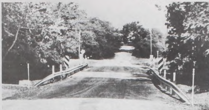
The bridge on West Eddy Street was opened last week after the Texas Department of Transportation accepted the project and gave the bridge back to the city of Muenster. Construction on the bridge began in March, but the street was closed to thru traffic in April 1999, when it was declared unsafe. Photo by Janie Hartman
