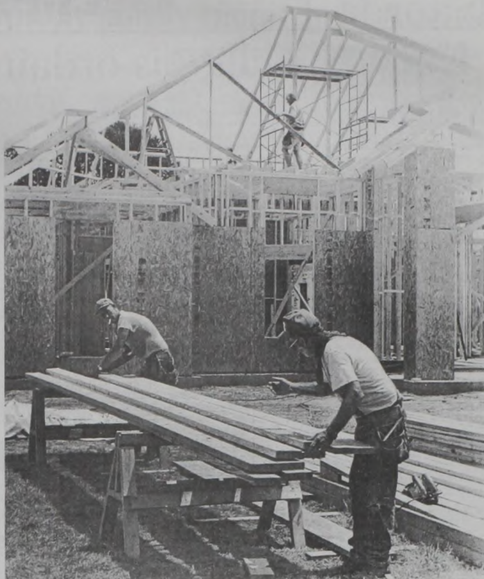
Construction is in progress in and around Muenster, including the future home of the Kenny Rohmer family, being built by the Rick Reynolds Construction crew. Janie Hartman Photo
