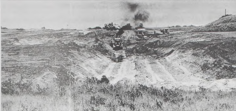
Work is progressing at the site of Muenster Lake as equipment digs out the "back drain" of the dam.
