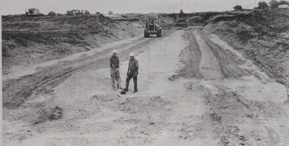
Bob Bauer (left), contracting officer and president of the Muenster Water Board, and project manager Raymond Lee of the NRCS check the progress at the site of the future Muenster Lake. Phase I of the construction continues as workers bury the foundation drain and begin raising the dam. Photo by Janie Hartman
