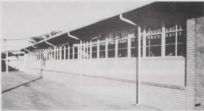
The Lindsay Junior High classroom north wall received a facelift and cleaning as part of the School Board's emphasis on maintenance and preparation for back to school. Dave Fette Photo
