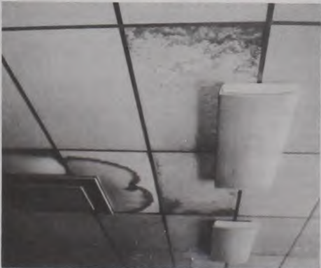
This water-damaged ceiling is just one of the maintenance concerns being addressed by the Lindsay ISD Board. Although there are many replacement ceiling tiles on hand, no action has been taken toward repairs. Courtesy Photo
