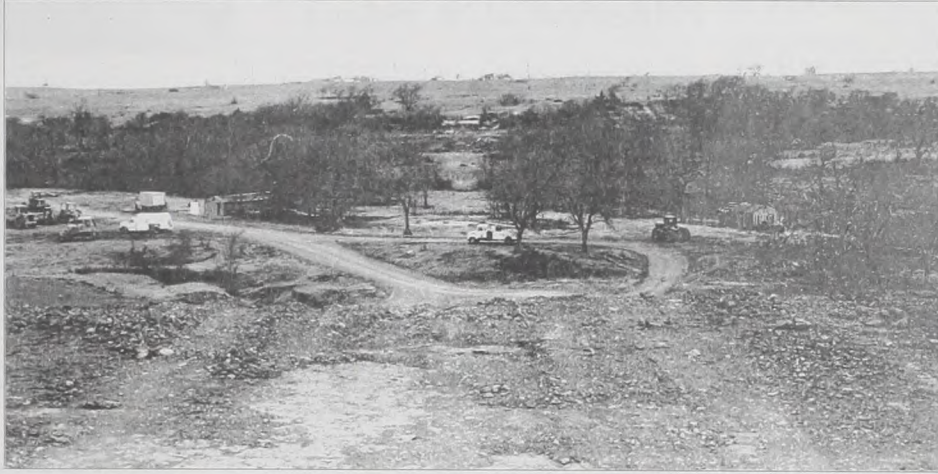
Phase 2 of the Muenster Lake construction awaits government funding to complete the dam. From the top of the
