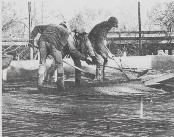
Soon to be home for bands, concerts, plays and all kinds of group functions, the new performing arts stage in Muenster's City Park is now a concrete reality. Dangelmayr Brothers Construction, at left, Chris Dangelmayr, Eric Walterscheid and Darrell Dangelmayr, poured cement Monday morning assisted by Ron Dangelmayr, Adam Wolf and Charles Knabe. The 48 foot wide stage will be covered and ready for Germanfest. Janie Hartman Photo
