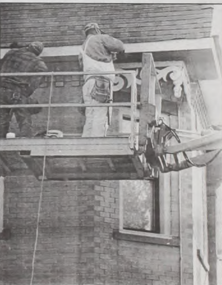
Work on the renovation of the Sacred Heart rectory is in full swing. Scott and Bert Walterscheid work on outside trim under the roofing on the north side of the house Wednesday afternoon.
