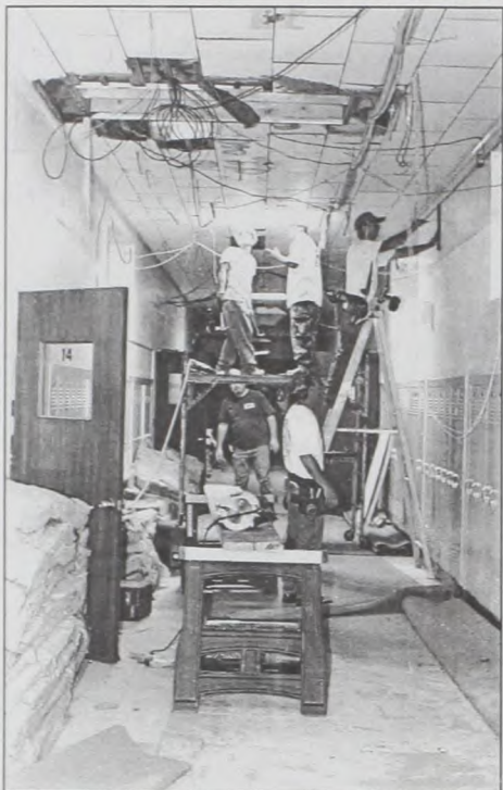
Work continues in the Muenster Junior High School building, part of the recent bond package. Improvements include replacing the roof over the west classroom wing, replacing heating, ventilation and air-conditioning systems and duct systems. Other improvements include an electrical upgrade, the replacement of the dropped acoustical ceiling and gymnasium roof and adding a fire alarm system to the complex. The MISD board of trustees met Wednesday night to also consider replacing the roof of the band hall. Janie Hartman photo
