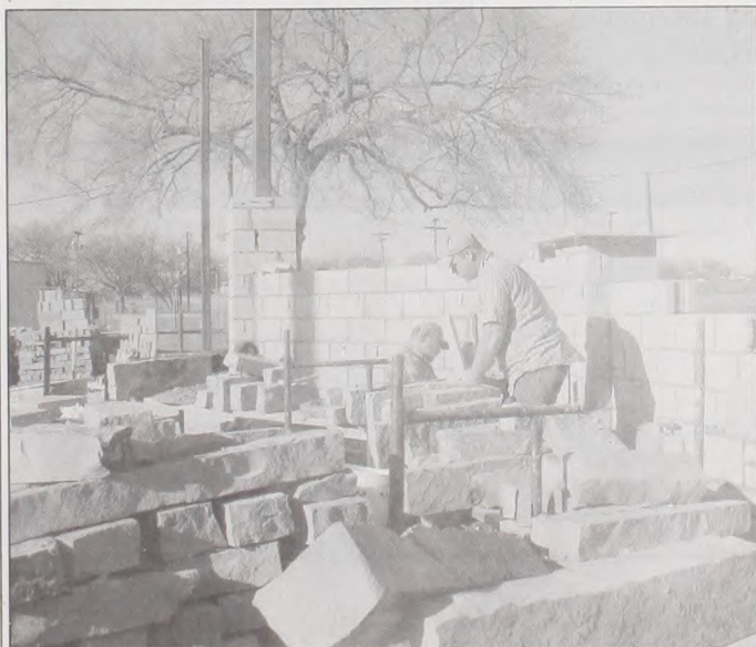
The Muenster City Park is receiving a much waited for entry way. Mike and Jake Hofbauer were building the entry wall this week in preparation for the new metal archway. Photo by Janie Hartman
