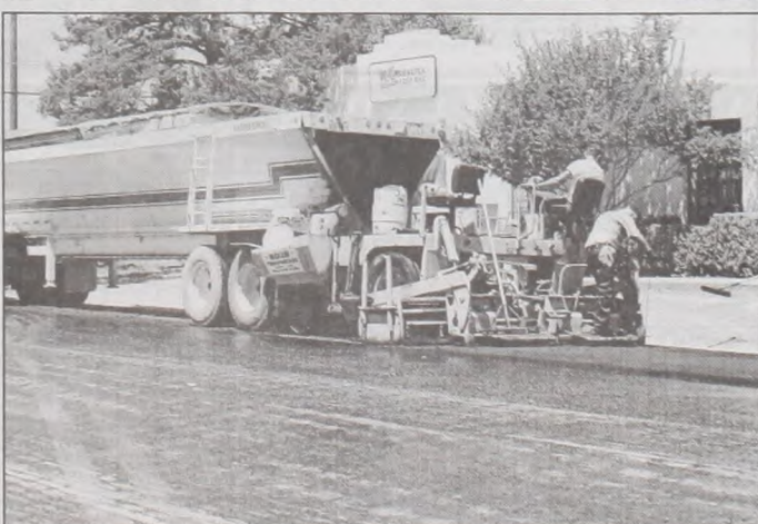
The City of Muenster has a major paving project underway. Five streets, First, Fourth, Seventh, Maple, and Sycamore are all getting a new hot mix surface. The contractor is seen here working on First Street. The top picture shows the finishing work on the second block, with the mix being put down on the 100 block in the bottom photo. Janie Hartman photo
