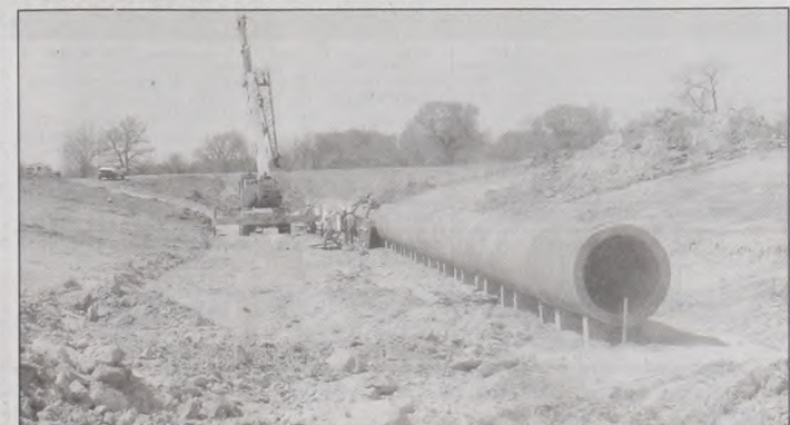
Phase II construction of the dam for Muenster Lake is in full swing. Above, the principle spillway is being installed. The 512 foot pipe runs the full width of the bottom of the dam. The insert workers pour concrete around the section. Janie Hartman photos
