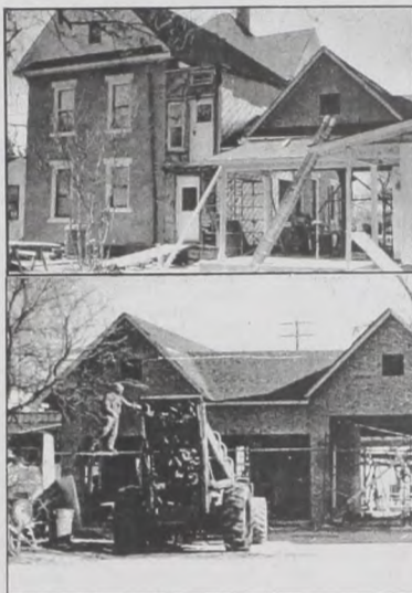
Progress continues on the Sacred Heart Rectory, as the original 1907 building gets a face lift and the new
