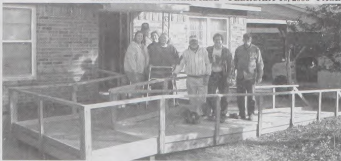
The Muenster Kiwanis Club united with the Dallas Ramp Project to build a wheelchair ramp for Paula Fleitman this past weekend. The Dallas Ramp Project builds approximately 200 ramps a year free of charge for the elderly and disabled. Generally they join forces with a local non-profit organization and provide the materials and know-how for the ramp construction; the non-profit organization provides the man-power. Pictured, from left, Jan Marion (daughter), Gus Fleitman, Melinda Cameron (daughter), Paula Fleitman, Dan Hamric, John D. Bartush, Mac Hopkin (not pictured Peter Heinkel and Don Emrick). Courtesy photo
