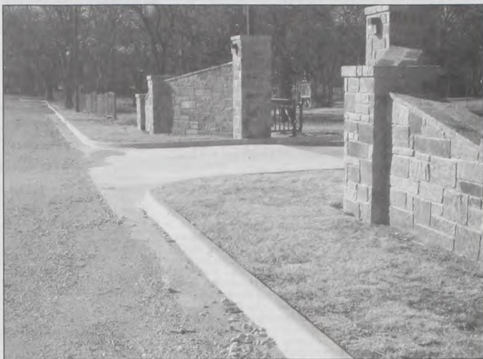
The above picture shows some of the progress made by City employees on the City Park refurbishment project. The curbing of driveways through the park has been completed. Janie Hartman photo
