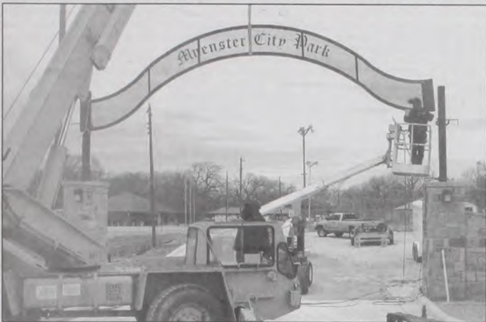
The archway entrance to the Muenster City Park neared completion Friday morning, as David Flusche, Jr. and Shawn Flusche of Structures, Inc. set the arch into place. The park entry, an improvement project of the City, was constructed at the request of Jewel Otto of the City Park Board. The all metal arch was designed and built by Neal Flusche of Flusche Enterprises.
