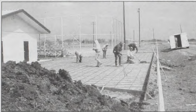
Dangelmayr Construction Inc. prepared a Handicap parking/dropoff location at the Muenster Jaycee ball complex earlier this week. Expenses on ball park improvements are paid for by Muenster Jaycee fundraisers, including the Raffle Dance, which will be held May 20. See any JC member for tickets.
