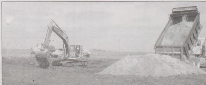
Work on the EMS western substation east of Muenster was in full swing this week as major dirt work began. County workers started with the station's foundation base. Janie Hartman photo
