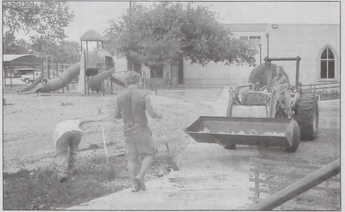
Workers put the finishing touches around the new playground equipment at Sacred Heart Catholic School in preparation for the new school year. Deborah Wood photo
