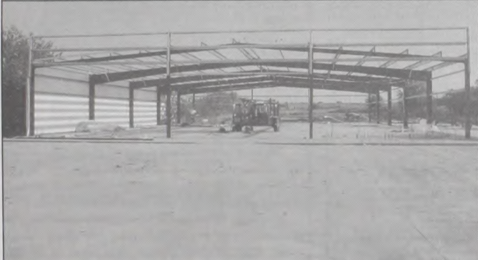
The construction is moving along smoothly on the new Dollar General store which is being built on the north side of Hwy 82 across from Bayers Kolonialwaren. Janie Hartman photo
