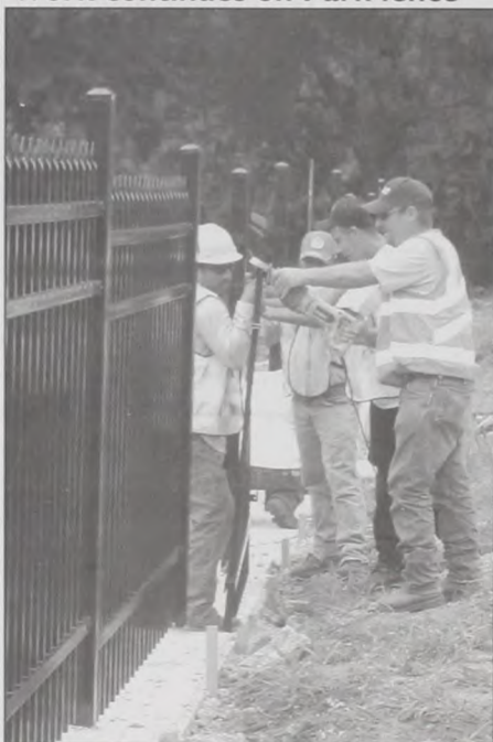
Workers of Marcom's Mowing Service are constructing the new fence along Highway 82 at the City Park, under the direction of TxDOT and Keep Muenster Beautiful. Janie Hartman photo
