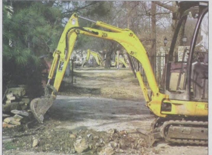
Spalj continues digging around town in order to install fiber optic lines to homes and businesses. The new lines will replace existing phone and television cables and allow for advanced voice and data services in Muenster. Janie Hartman photo
