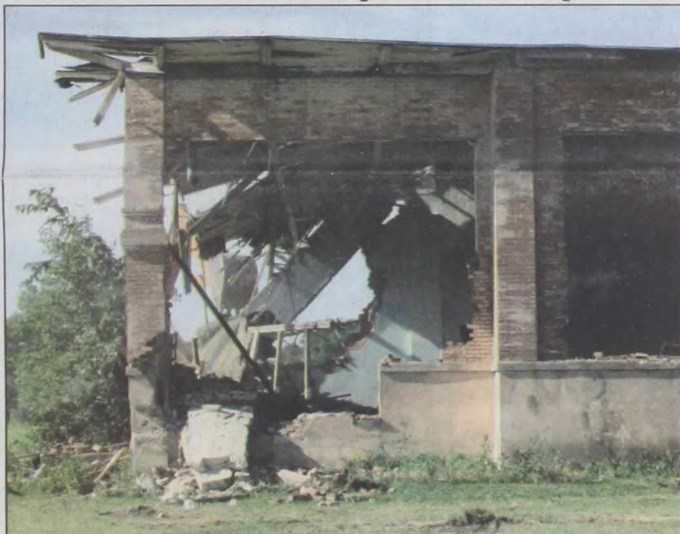
Built in 1912, the original Myra school building was knocked down to a pile of rubble Monday morning. The Myra Volunteer Fire Department will construct a 60x60 fire station with four truck bays in this location and use the "add on west classrooms" for meetings and community events. Shown is the northeast corner where the cornerstone was recently removed. Janie Hartman photo
