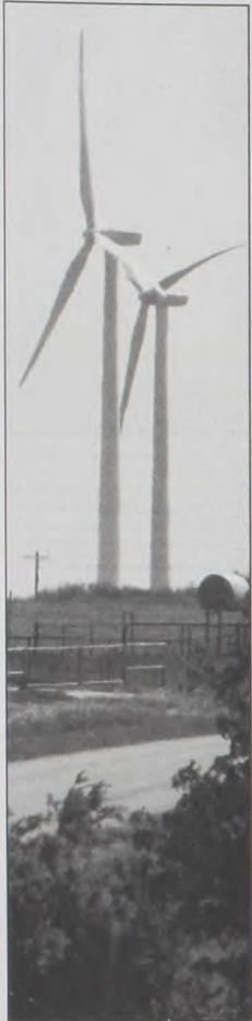
Two of the 75 wind turbine generators being installed by FPL Energy. Janet Felderhoff photo
