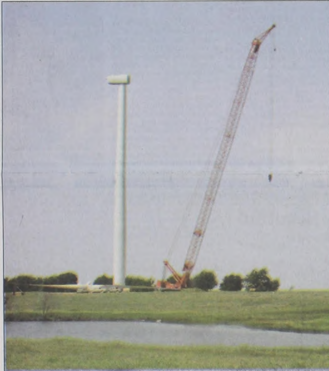
There is a new look to the skyline north of Muenster as Wolf Ridge Wind, L.L.C.'s wind turbine generators are in the process of being erected. Several turbine towers have been standing for a while, but last Thursday, the first glimpse was had of what they look like assembled. Above - the tower with nacelle atop awaits the blade assembly. The blades are assembled to the hub on the ground (see bottom left of photo). The whole unit is lifted by a crane measuring 330 to 340 total feet in height. The crane's boom is 314 feet long. Photo at right shows massive size of crane being used. Each of the three wind blades measures 132.2 feet in length. Total height is over 400 feet for the wind turbine generator. Each WTG will power 400 homes and when all 75 WTG are operating they can power 30,000 homes. They will generate electricity at wind speed as low as 8 m.p.h. and up to 55 m.p.h. The optimum speed is 25 to 35 m.p.h. Janet Felderhoff photos
