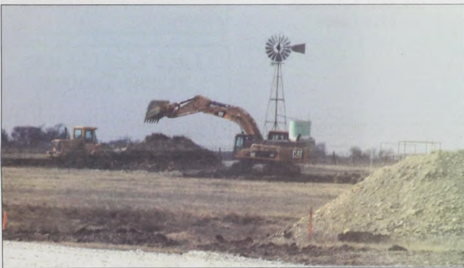
Work has begun and continues on the site of the Wolf Ridge Wind Energy Project north of Muenster. The construction of roads can be seen cutting through pastures along with the building of fences and gates. Also, a lay down yard will be located on CR 430 with a
