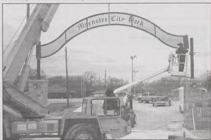
The archway entrance to the Muenster City Park neared completion in early March. David Flusche, Jr. and Shawn Flusche of Structures, Inc. set the arch in place. The park entry, an improvement project of the City, was constructed at the request of Jewel Otto of the City Park Board. The all metal arch was designed and built by Neal Flusche of Flusche Enterprises.
