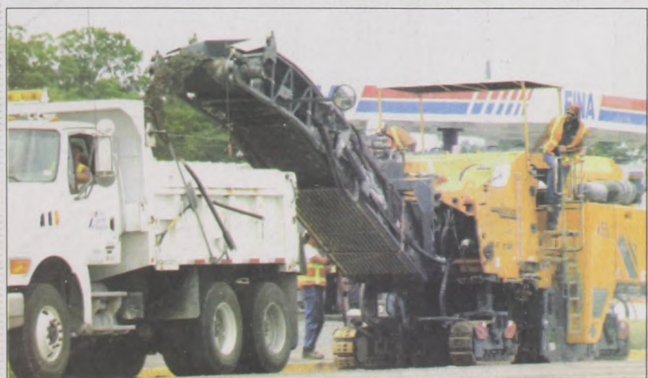
Crews from the Texas Department of Transportation began work this week on Highway 82 through town, peeling off the paved surface. The project started last summer, but the surface did not stay in place, causing holes and bumps that have been patched and covered the last year. Hopefully, this finished job will give travelers a smooth ride through Muenster.
