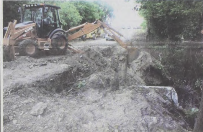
Precinct #3 workers replaced a 35 year old culvert on CR 300 this past week. A 6 foot diameter, 50 foot long, corrugated culvert was placed in the 20 foot deep hole. Resurfacing the road and adding railing will complete the project. Janie Hartman photo
