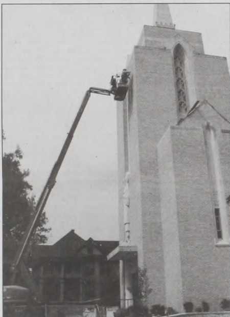
Work continues at Sacred Heart Church, including the replacement of mortar, as shown, and roof repair. Janie Hartman photo
